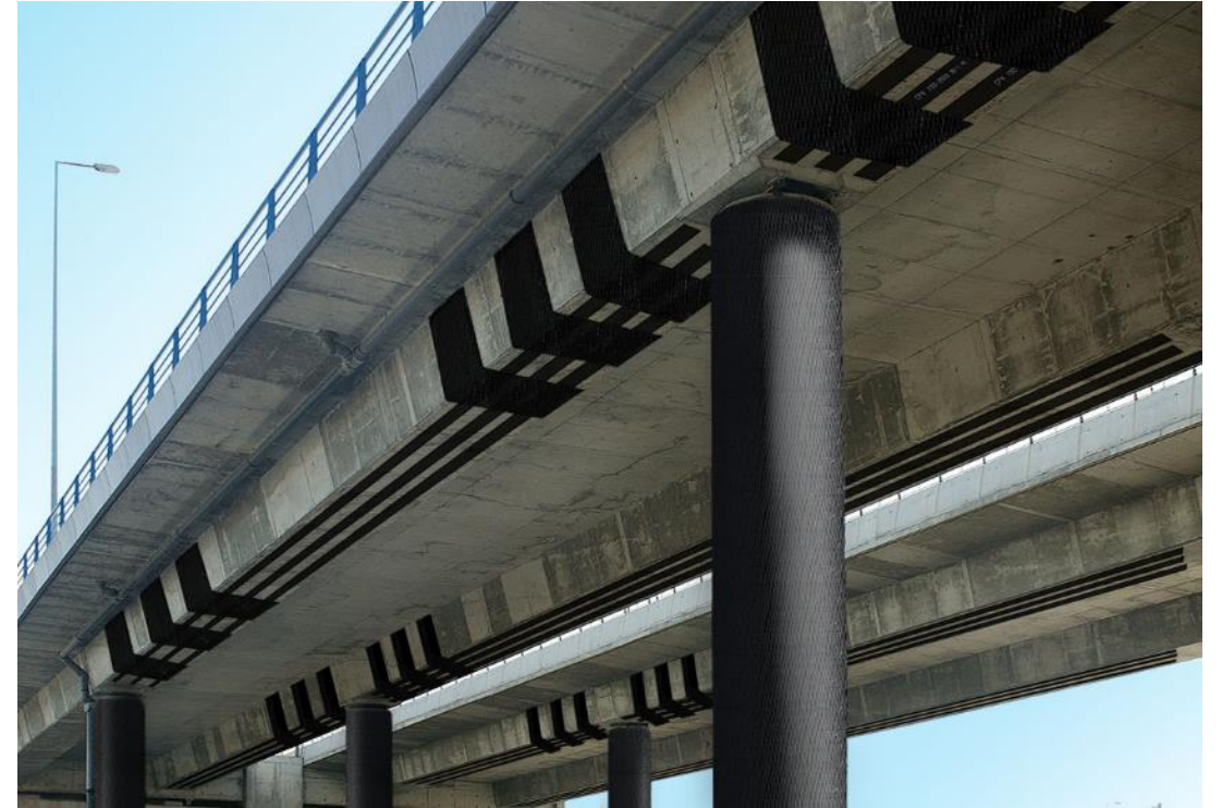
Example of a bridge with girders supported by CFRP and columns wrapped in it.
